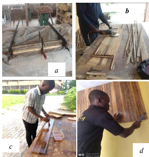
Plate 4. Panel Production and Installation Processes (a) Clamping (b) Sanding (c) Finishing (d) Installation
